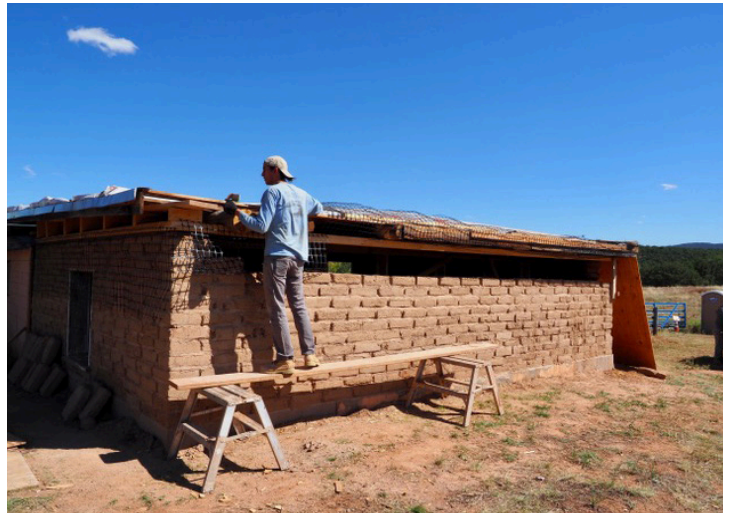
Training at the Forked Lightning Ranch Stable Restoration, Pecos, NM included adobe-making, foundation repair, structural bracing, wall building, stitching, window and door repair and plastering. (right)
