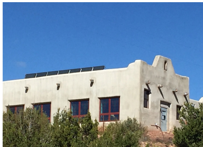
Ribera Rooftop Solar Installation (courtesy image)
