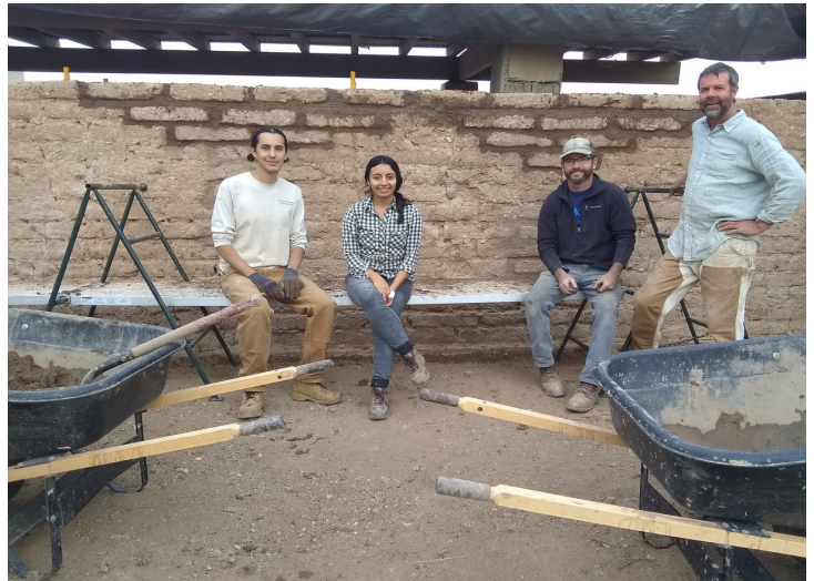
Workshops restoring Civilian Conservation Corps adobe walls occurred at Casa Grande Ruins, AZ. (below)
