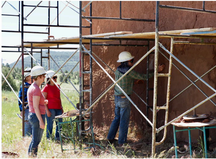
Buena Vista and La Cueva churches in Mora, NM hosted adobe preservation workshops for volunteers and interns. (above)
