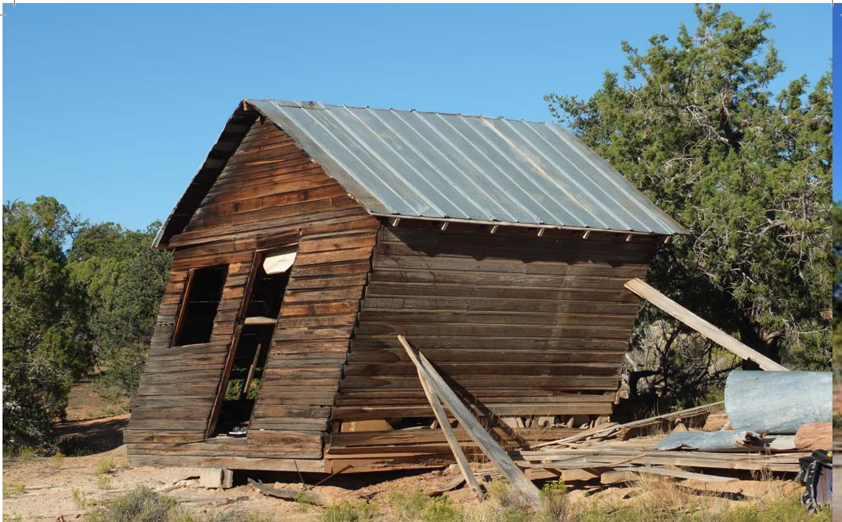
Left Photo: Before Stabilization Workshop Right Photo: After Stabilization Workshop French's Cabin Glen Canyon, UT
